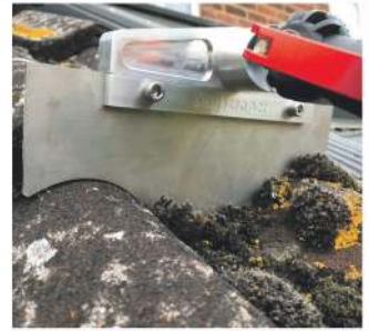
Moss Removal with Skyscraper
